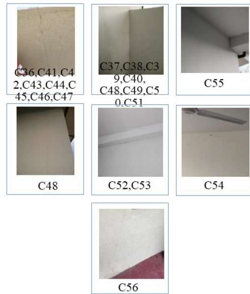
Fig. 5. Second floor cracks
