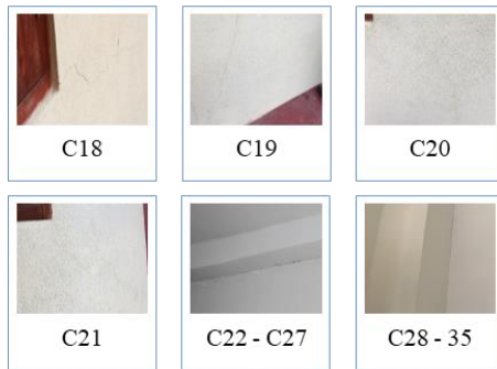
Fig. 4. First floor cracks
