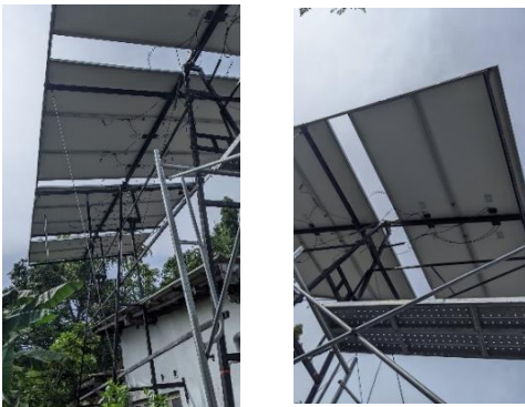
Figure 9 – Solar Panel Structure
