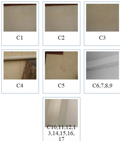
Fig. 3. Ground floor cracks
