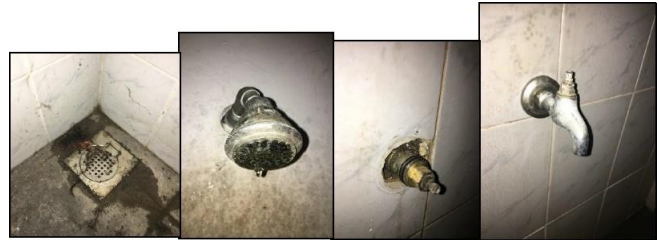
Fig. 1. Blockages, Leakages and Damages
